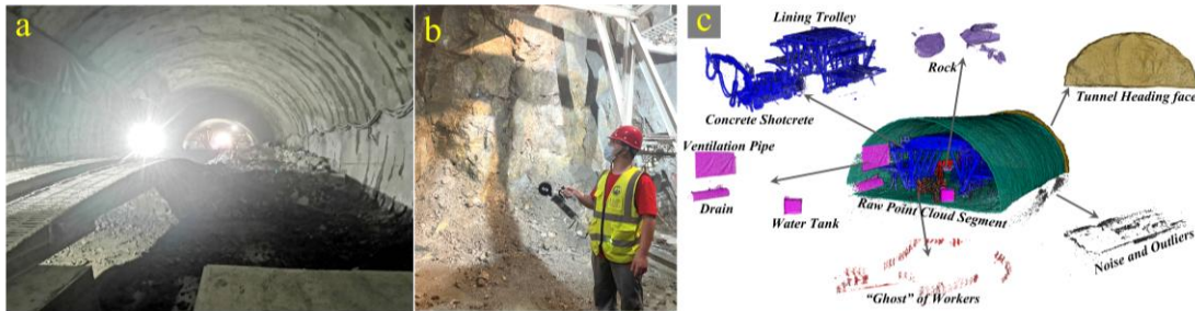
Figure 1. (a) The tunnel construction site; (b) Tunnel 3D point cloud data is being collected using HLS on the site ; (c) Complex point cloud data of tunnel construction site (Cui, 2023).
